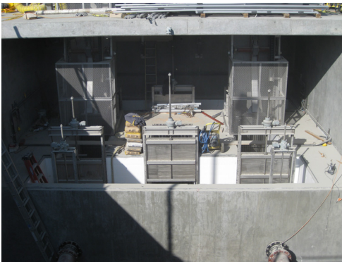
Figure 5 - New sewage clean-out system
